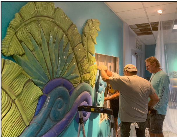
De-installation of the airport's public art in preparation for construction of the new terminal.
