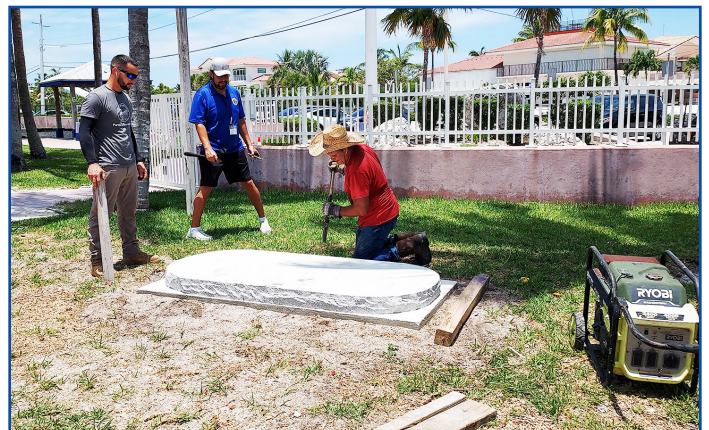
City of Marathon’s crew assist in laying the foundation for the new artwork.
